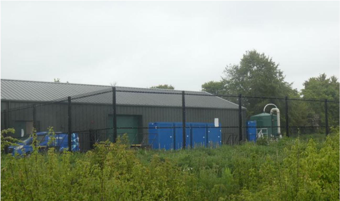
The large green denitrification plant and chemical storage at the Oughtonhead pumping station
